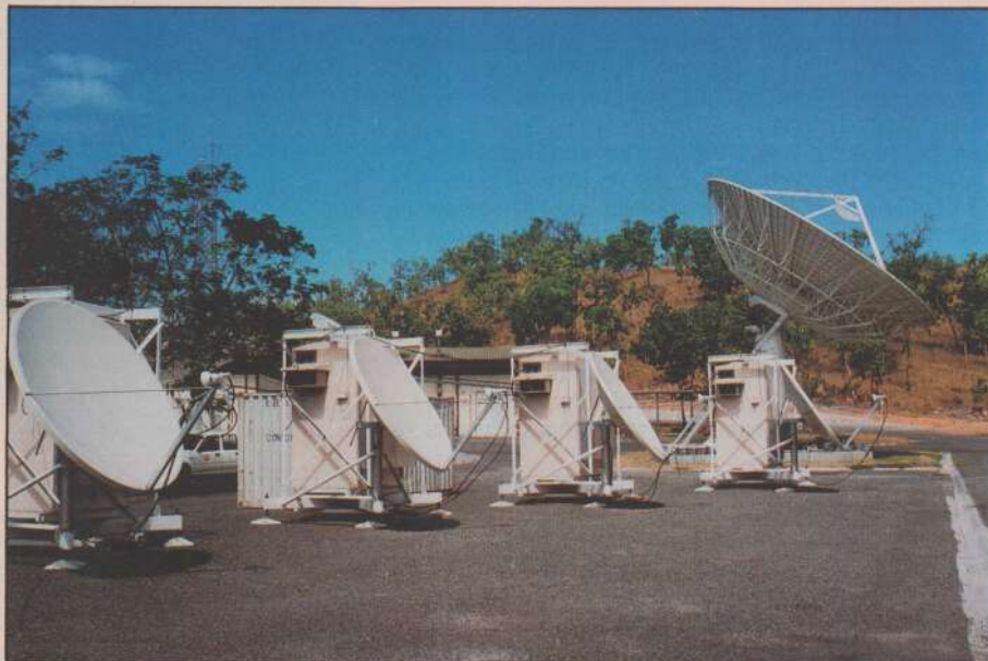
Four transportable interim mobile earth stations installed and ready for use in emergencies. In the background is the full DOMSAT Earth Station
