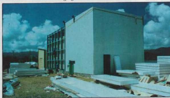
Help at hand: the new ice plant at Pohnpei
