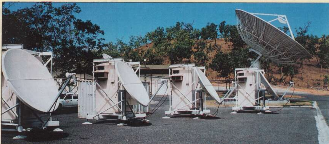
Advanced technology: four transportable interim mobile earth stations installed and ready for use in emergencies. In the background is the full DOMSAT Earth Station
