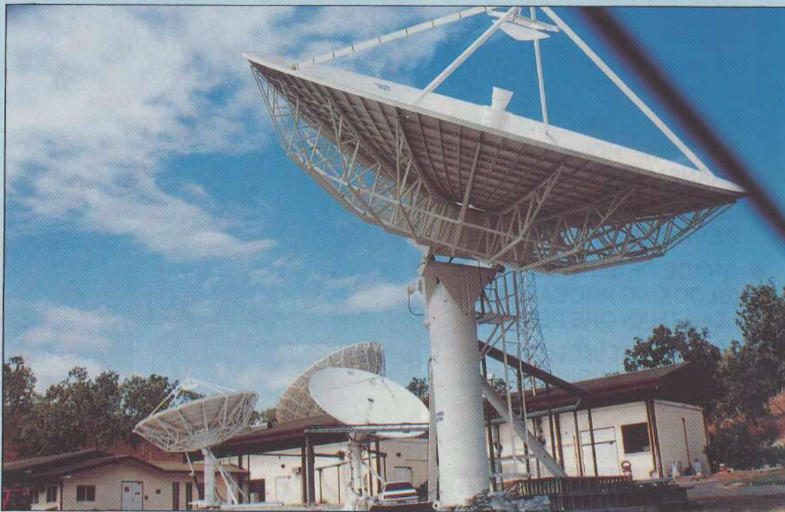
Earth Station: the full DOMSAT station with the interim DOMSAT (centre) and the Optus earth station at left
