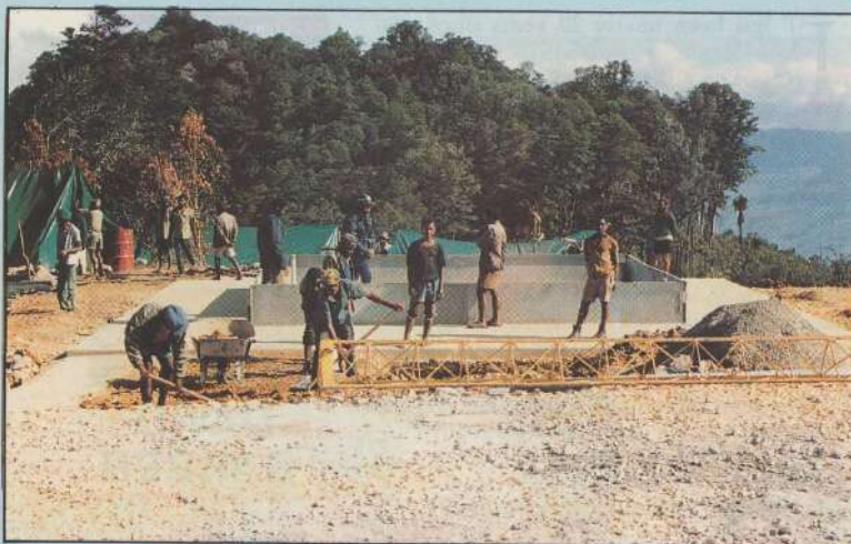
Southern Islands Province: site for a new repeater station
