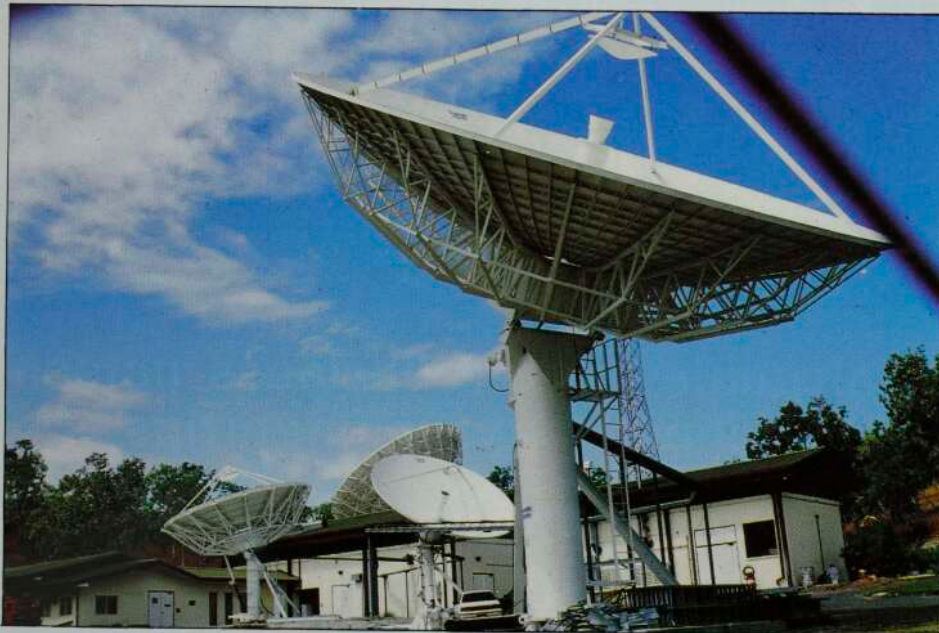
The full DOMSAT earth station in PNG: with the interim DOMSAT (centre), Optus earth station (left) and standard "A" Intelsat earth station in the background.
