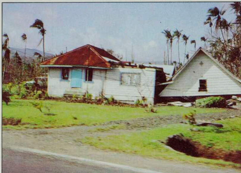
Misplaced roofs: the rest of the home fared a little better
