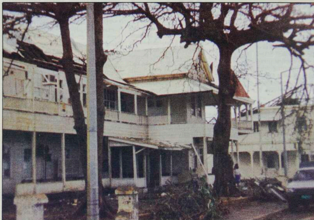
Battered: the historic government buildings and many records were damaged
