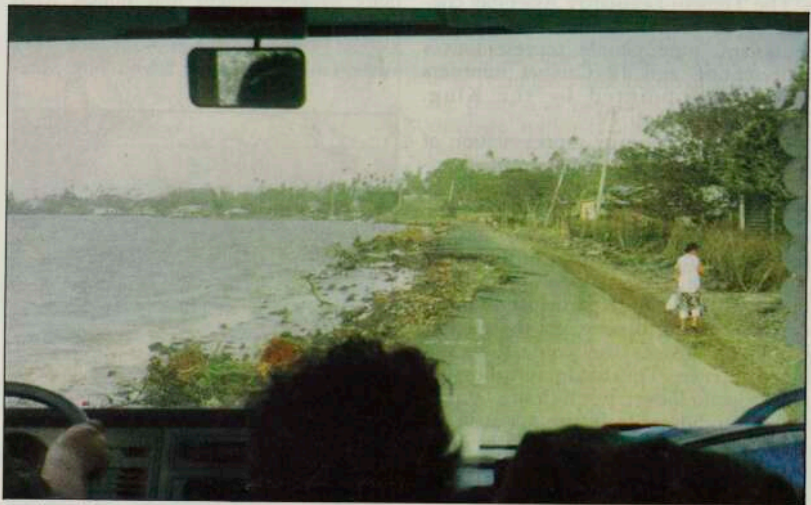
Destruction: strong waves peeled away the tarseal of this road near Apia in Western Samoa.
