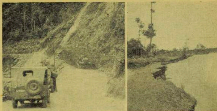
These photographs show something of the problems of maintenance on the road between the New Guinea coast, at Labu, and Wau, about 90 miles inland. On the left, a bulldozer is clearing away a slip; and on the right the Markham River has eaten into the road formation. Only by the efforts of the gold-mining companies, Bulolo Gold Dredging, Ltd., and New Guinea Goldfields, Ltd., is the road kept open to traffic.
